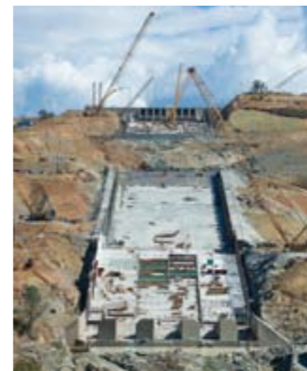
Photo of the primary spillway at Oroville Dam on September 22, 2017, under construction as part of the recovery project in response to the February 2017 incidents (photo courtesy of California Department of Water Resources).
